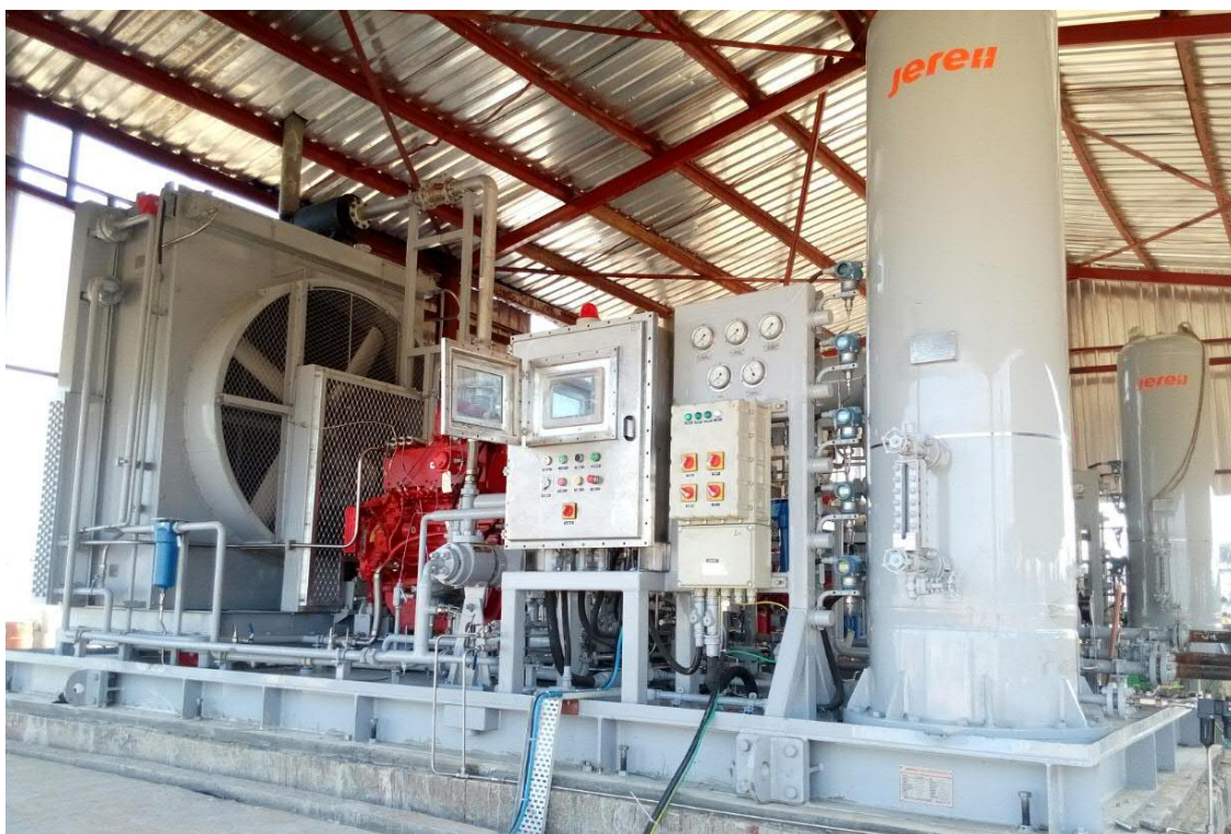
Jereh compressor in Nigeira
